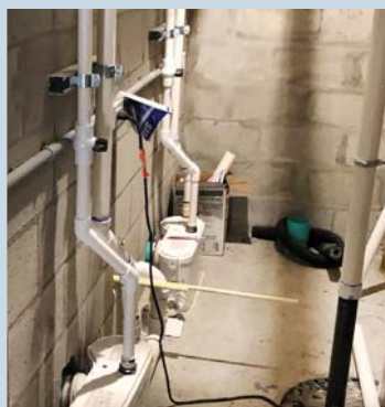
Sanibest Pro grinder units installed to discharge the wastewater from three toilets and a urinal.
