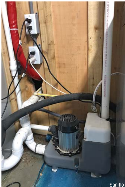
The Sanicom 1 unit installed to discharge the gray water from three hand-sinks and three tub-dishwashing sinks in the bar area. The unit's 1-inch discharge pipe (top left) runs eight feet vertically and connects to an existing wastewater line.
