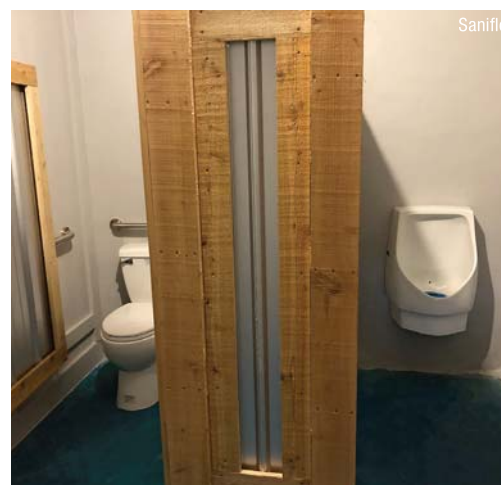
A urinal and toilet are connected to a Sanibest Pro in the men's restroom.
