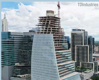
Block 185, still under construction, is attempting to achieve a LEED Gold Rating under LEED v4 for BD+C: Core and Shell.
