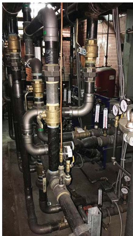
Tight confines, high temperatures and tricky pipework were just some of the challenges facing First Service Mechanical.
