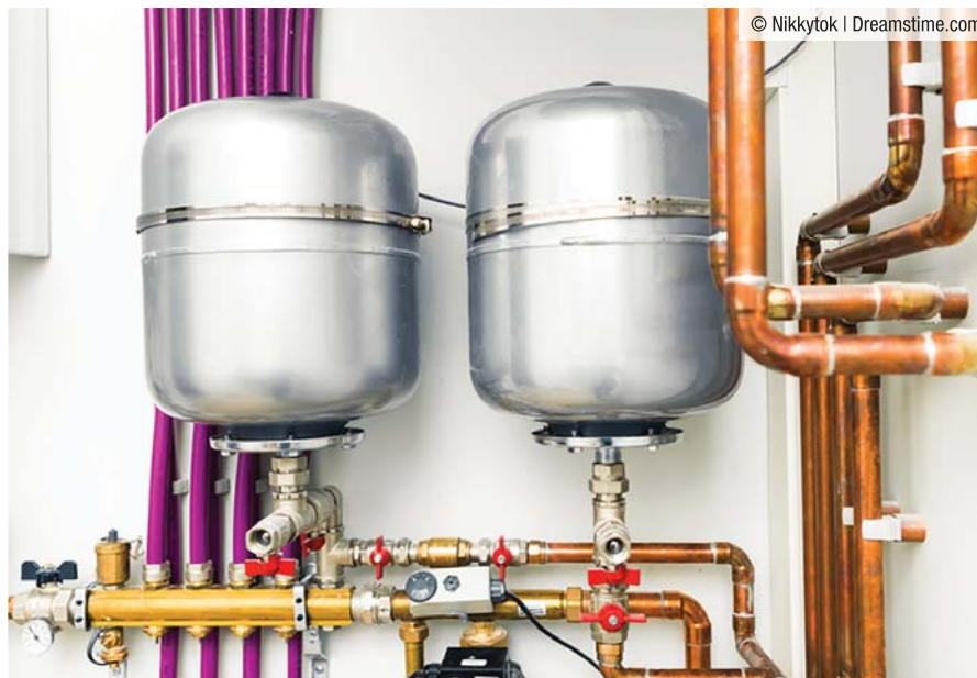
Expansion tanks in boiler-room.
