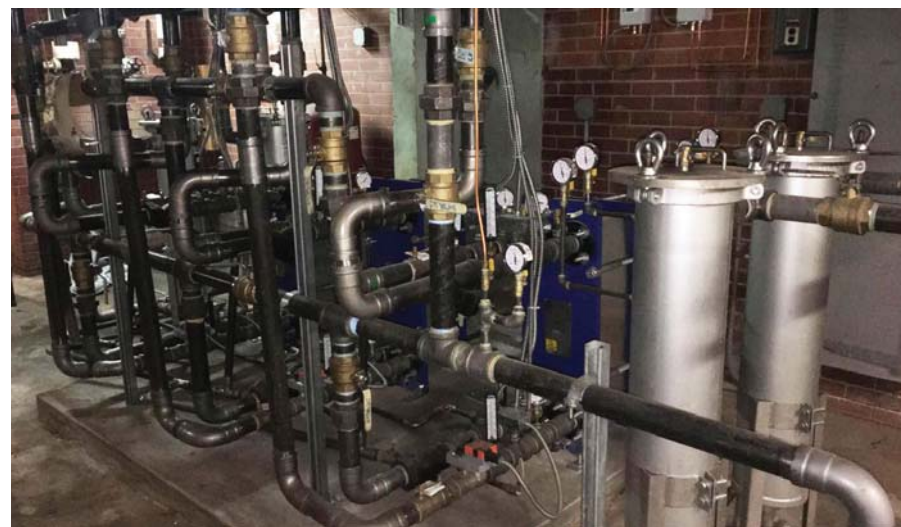
Another view of the mechanical room at St. Joseph Villa.
