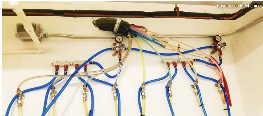
Glycol piping and tap lines at the Oasis Bar in Sturgis.
