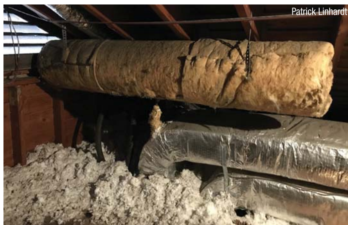
The mystery expansion tank is discovered at last.
