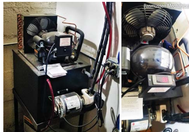
The chiller pump and thermostat.
