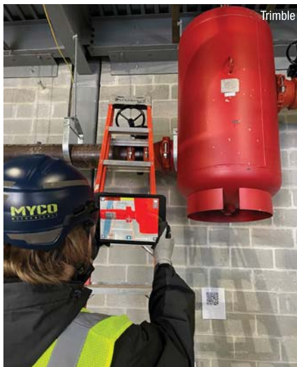
A Myco Mechanical technician verifies equipment placement using the Trimble AR system.
