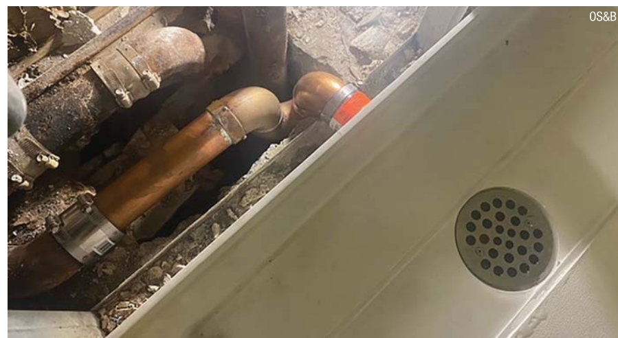
Top view of shower pan showing drain cover installed- Cover palte is polished chrome but still has plastic protection sheet on it.
