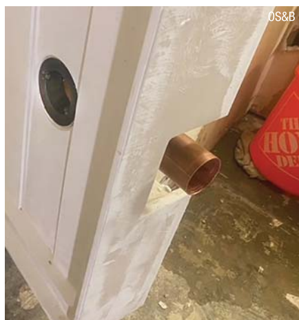
Side view of shower pan showing the side discharge shower body with brass pipe attached.
