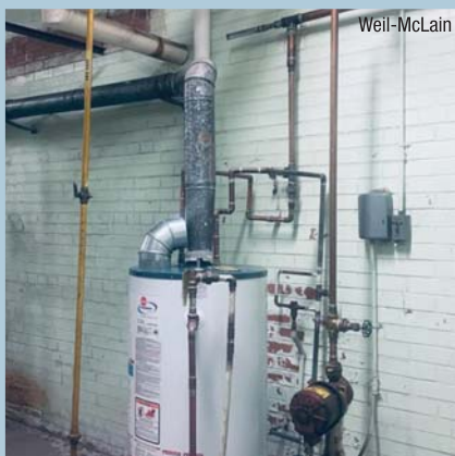
Part of the old system before the upgrade.
