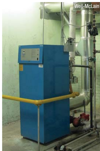
The old boiler before the upgrade.
