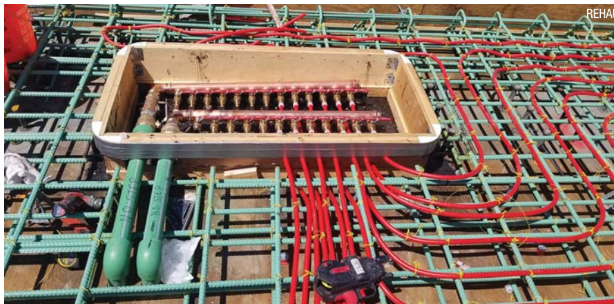
Frailey fabricated seven 2-in. (6 cm) custom copper manifold vaults to house distribution piping, using F1960 fittings for connections to SIM loops.
