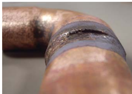
Too wide of a clearance between the two parts during brazing results in a gap that will cause joint failure.
