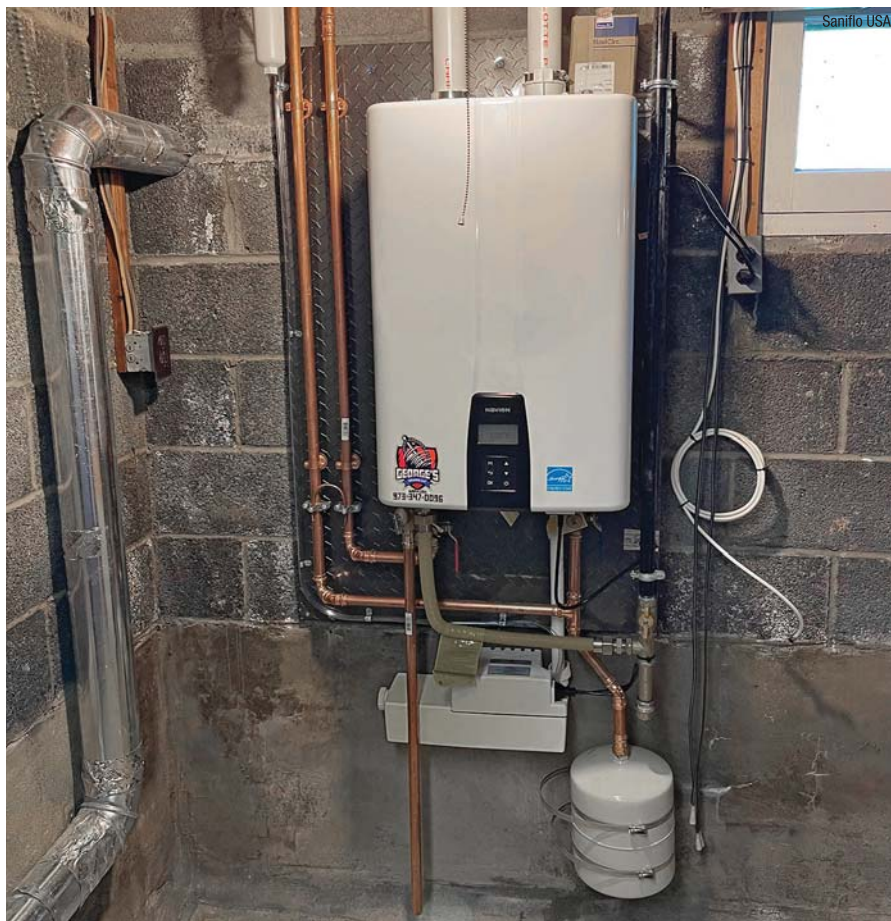
The finished tankless installation. The Sanicondens Best Flat unit can be seen underneath the Navien unit, just above the expansion tank.
