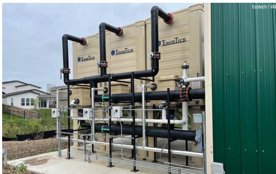
These are the auxiliary cooling towers connected to the GeoGrid to mitigate peak demand should they be needed.
