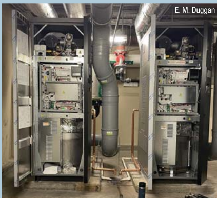
The original boilers at luxury condo building 100 Pier 4 in Boston needed to be replaced because of failing heat exchangers.
