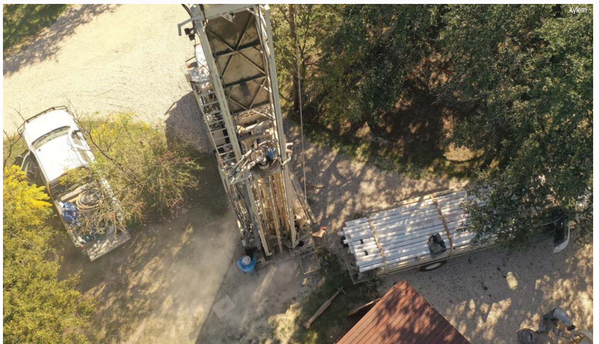
Hometown H2O, the partnership between Xylem, Waterboys and WaterWell Trust, installed a new well for the Solares family of Bertram, Texas in December 2021.
