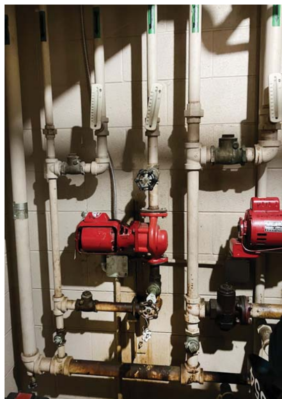
Two of the three pumps that were installed, all piped the same way.
