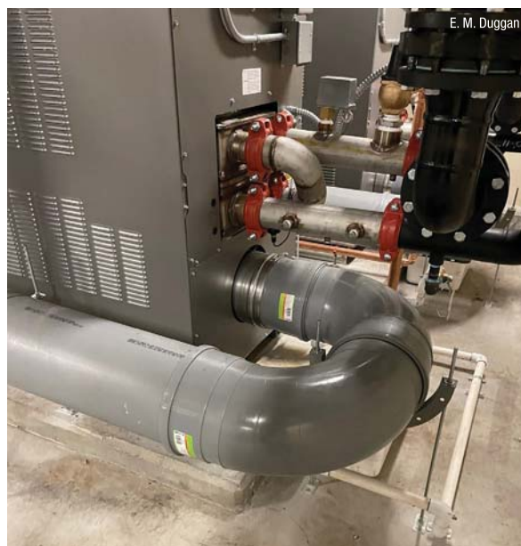
The Duggan crew removed the old flue and installed a new flue using Centrotherm polypropylene flue piping to meet code. John Lamb, account manager at Duggan Mechanical Services, notes that the plastic piping has fewer leaks than stainless steel.
