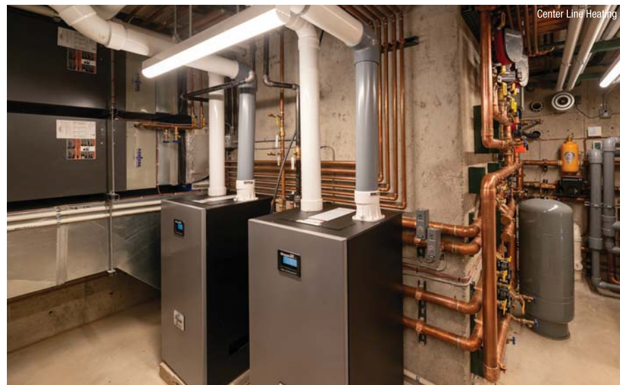
Center Line installed two, 399 MBH Aspen light commercial boilers for the snowmelt, radiant, pool heat and DHW.
