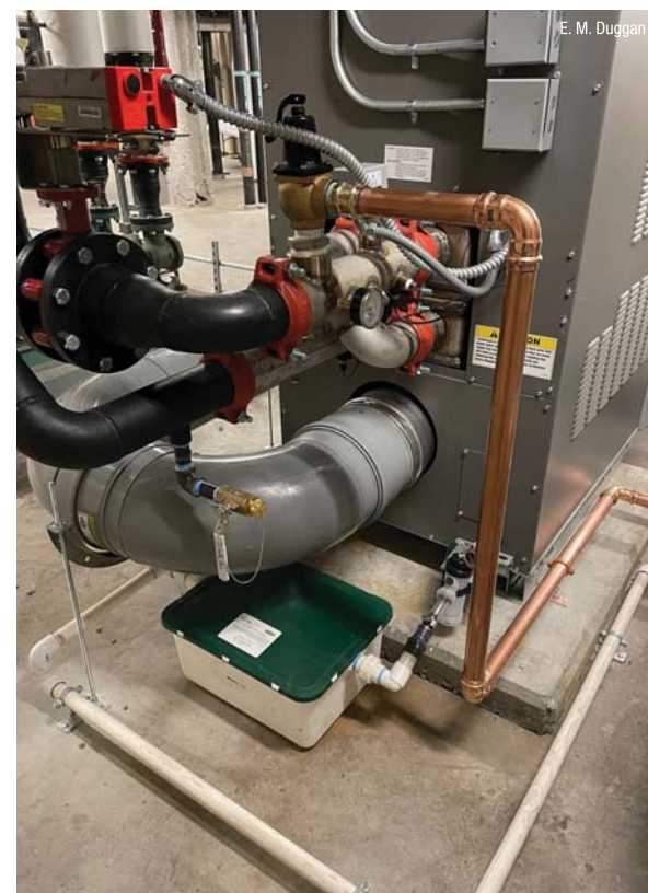
The new boilers serve the condenser water loop for in-unit heat pumps to the 369 luxury apartment units at Boston's Pier 4.
