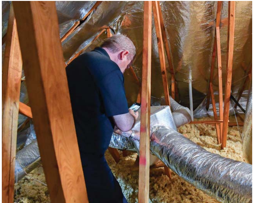
Ductwork that is properly sized and sealed helps defend against loss in the attic.
